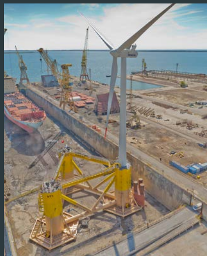
WindFloat 1 prototype ready for load-out at the Lisnave Shipyard in 2011. Picture shows the platform architecture including Water Entrapment Plates and the turbine sitting atop the right-most of the three columns Image courtesy of Principle Power
